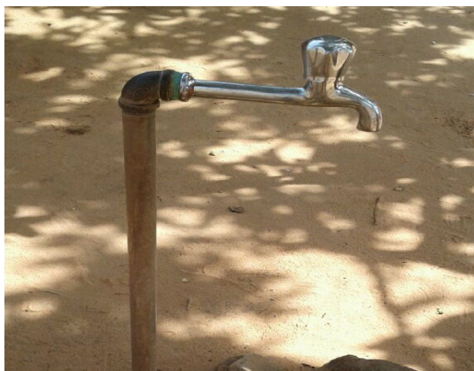
Yard pipped water
